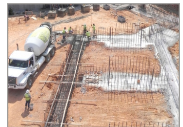
The construction progress of the new Bruno Cancer Center as of August 28, 2013
